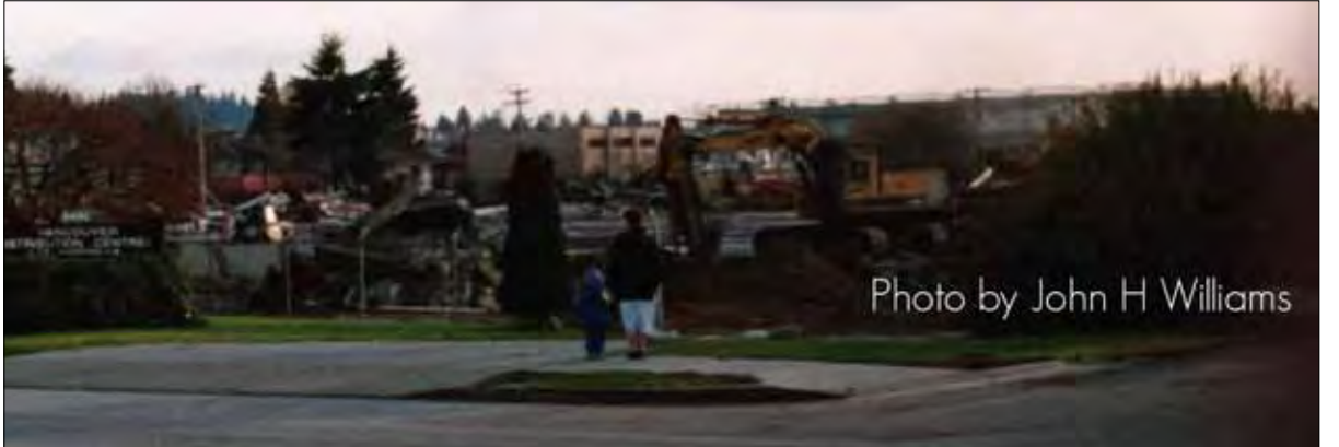
Loretta Houben and her young son watching the demolishing of the warehouses on Wellington Ave, 1992. Photo courtesy of John Williams.
